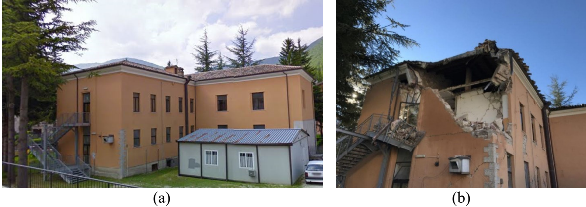
Figure 7: The corner mechanism activated in a masonry building during the 2016 Central Italy earthquake.
