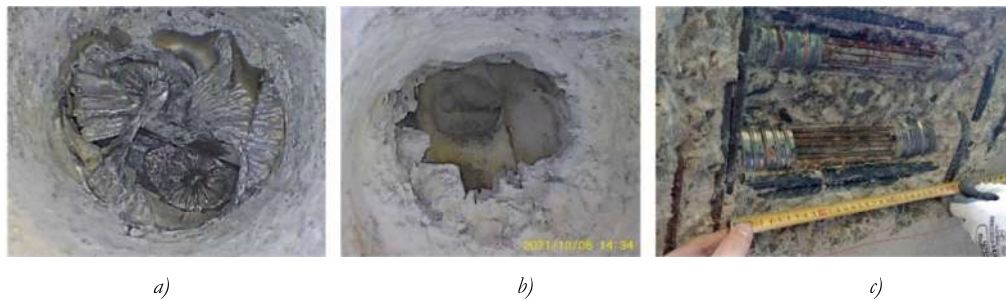
Fig. 3. A) Poorly executed endoscopy: the mashed duct does not allow a correct evaluation; b) well-executed endoscopy: there is no grouting inside the duct; c) exposed cable with evident corrosion phenomena.
