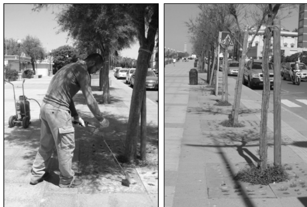
Figure 9. Trolley flaming machine at work (a) and an overview of the treated avenue (b).
