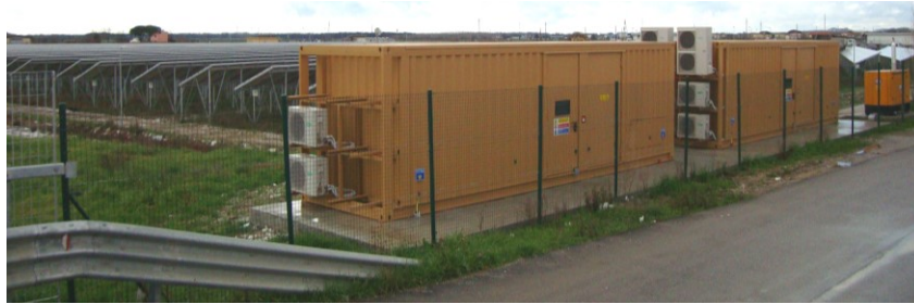
Figure 1: Picture of the inverter and storage containers
