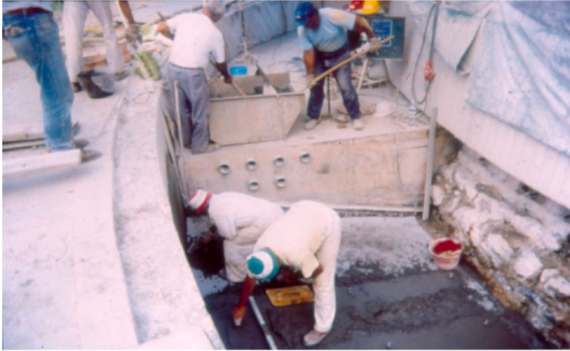
Figure 9. Construction of the northern sections of the ring beam for the ten anchors.
