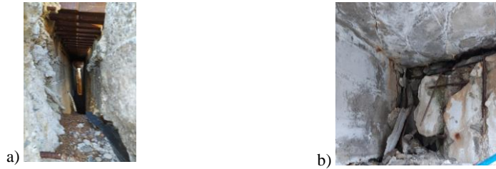
Fig. 3: a) Partial detachment of the deck from the right abutment; b) Progressive movement and locking of the deck toward the left abutment.
