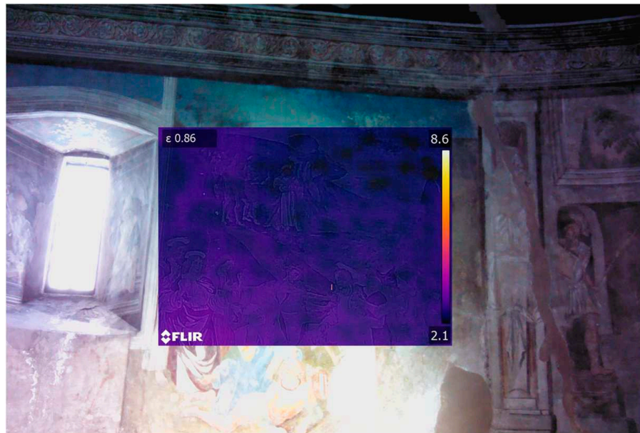
Figure 2. Example of passive thermography analysis used to identify the support wall texture. Stones with irregular shapes can be distinguished behind the fresco.
