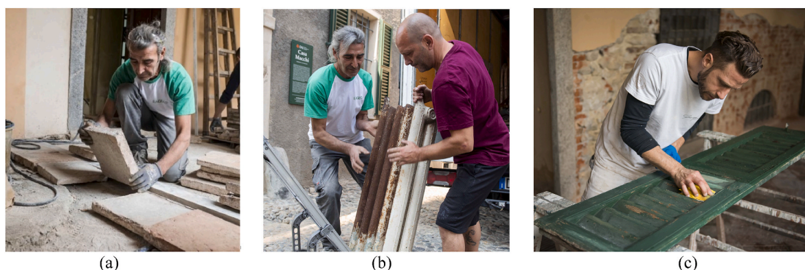
Fig. 7. Casa Macchi: restoration of (a) old roof tiles; (b) radiators, and (c) old wooden shutters (Source: FAI).
