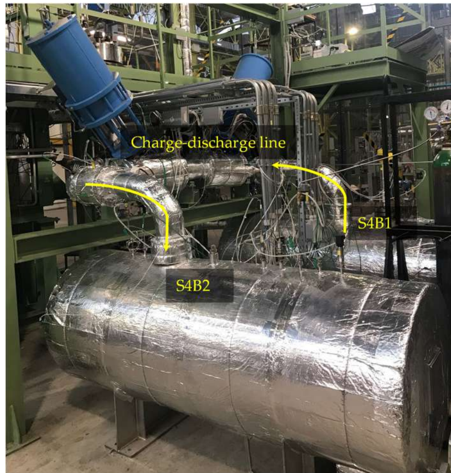
Figure 6. Storage (S4B1) and drain (S4B2) tanks, loading and discharge lines.
