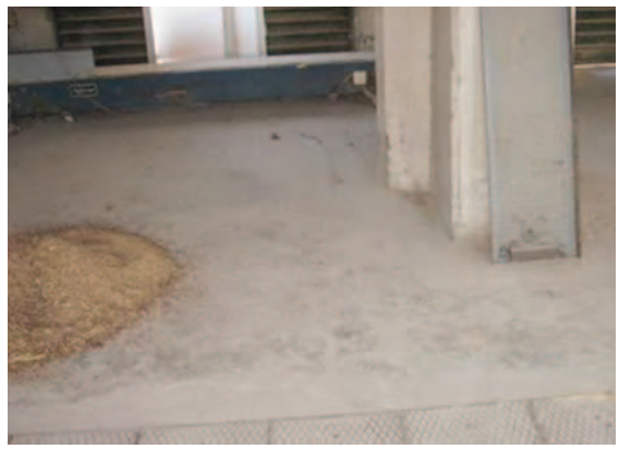
Picture 7: Detail of the flooring. Presence of several patina and cracks
