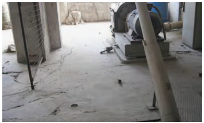
Picture 8: Detail of the flooring. Presence of several patina and relevant not cross cracks
