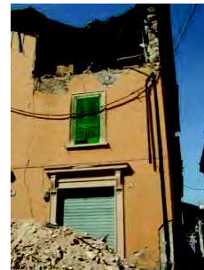
Figure D.2 Out of plane overturned wall
