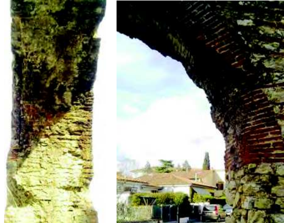
Arch n. 163 – Side A Deterioration at the intrados of the arch and deterioration of the façade of the arch
