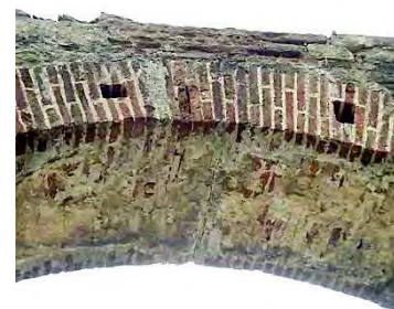
Arch n. 137 – Side A Detachment of some brick elements from the arch
