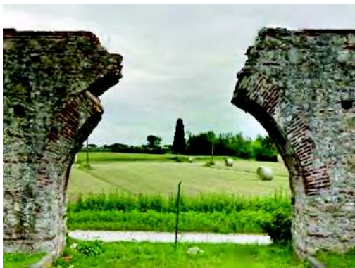
Arch n. 395 – Side A Partial collapse of arch
