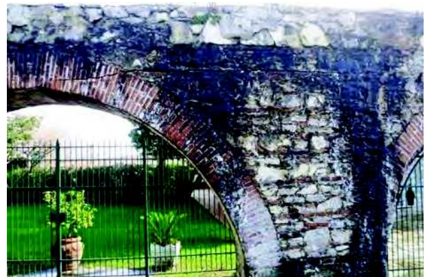
Arch n. 16, 17 – Side A Vertical settlement appearing by a crack in the backfill, extended to arch's brick
