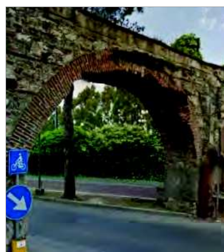
Figure 22 Arch n°162, damaged by vehicles impact
