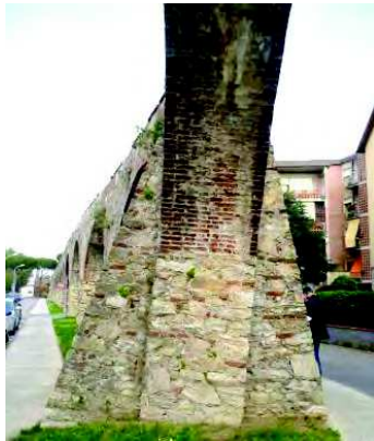
Arch n. 144 – Section Out of plane rotation (9°) of a pillar between buttresses
