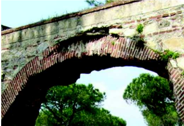
Arch n. 163 – Side A Deterioration of arch's bricks at the extrados and intrados, caused by lorry impact
