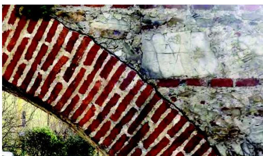
Arch n. 113 – Side B Detachment between the arch's bricks and the backfill.
