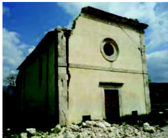
Figure D.1 Overturned tympanum and cracks indicating incipient overturning of the building facade
