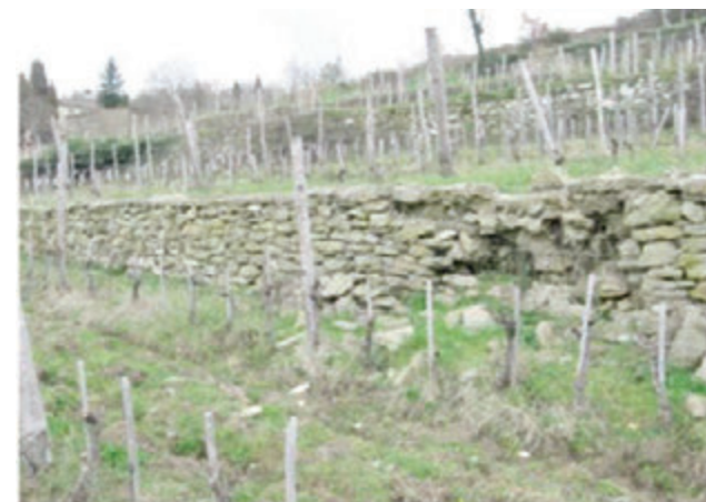
Figure 8. Surveyed terraced walls with slumps and erosion
