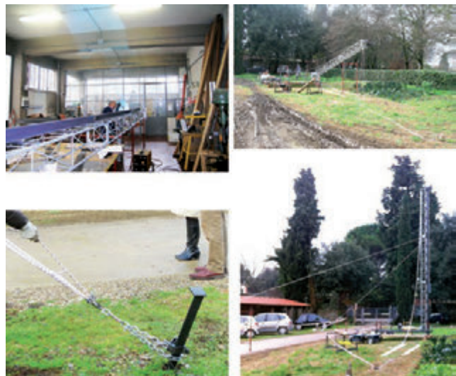
Figure 3. Pile driver under construction; uplifting; stays hooking system, and pile driver in working position.
