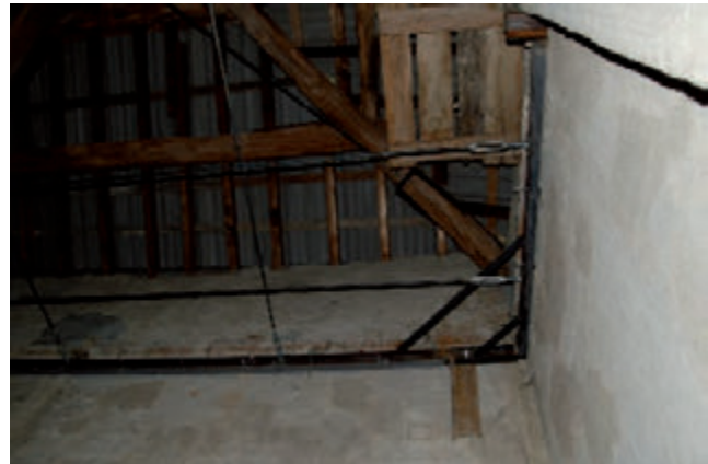
Figure 9. The loop created from inside: the U profile fastened to the masonry by the anchored pins, the triangular frame at the corner and the steel tie rods are shown.
