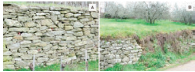
Figure 1. Terraced walls with an implemented drainage system (A), and effects of a failed maintenance (B).
