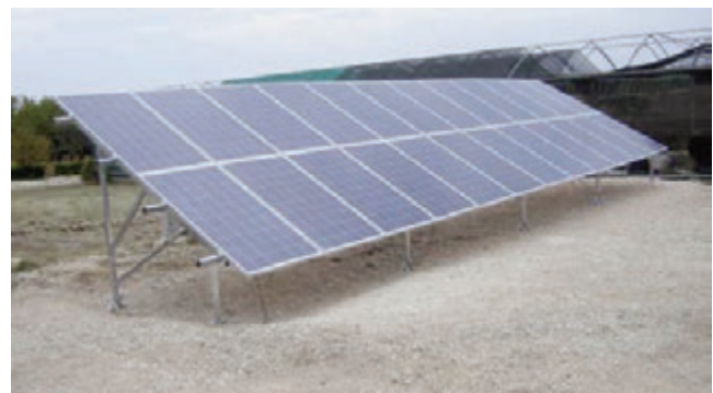
Figure 4. The photovoltaic array.
