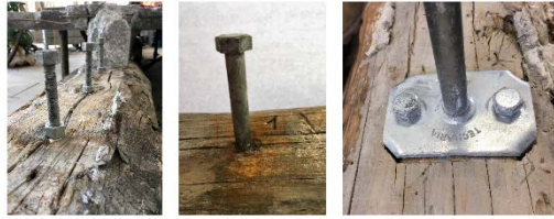
Fig. 7. Shear connectors after the test: (a) beam A, (b) beam B and (c) beam C.
