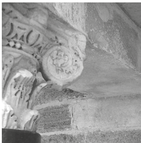
Figure 4 - Detail of the wall of the second loggia made up of prevalently calcarenite Panchina and one black limestone ashlar.
