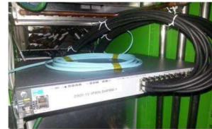
Fig. 14. The switch collecting all data links of a crate.
