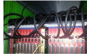
Fig. 13. CREAM data links to the switch.
