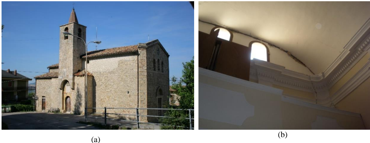
Figure 3: San Michele church: global view (a); incipient out-of-plane mechanism of the façade, view from inside the building (b).
