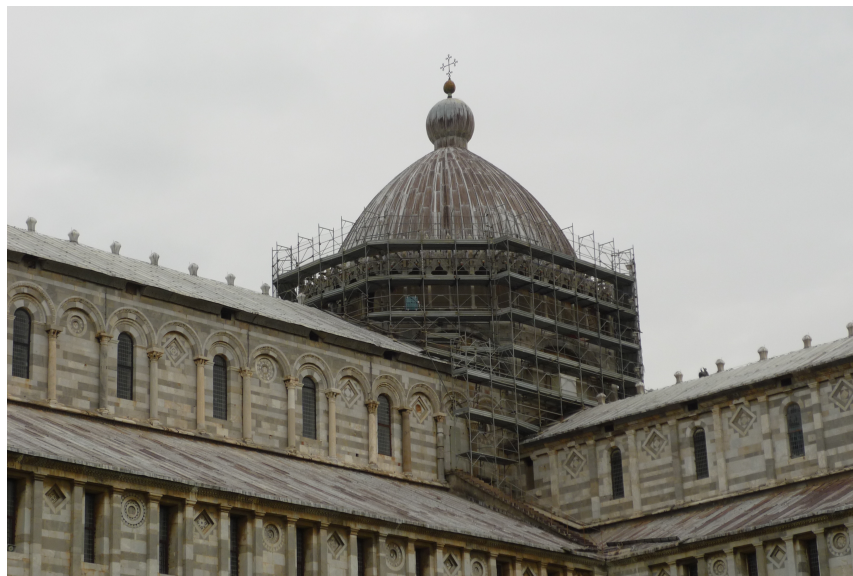
Fig. 1. The recently erected scaffolding for the restoration works, in preparation for the 900 th anniversary of the Cathedral dedication.
