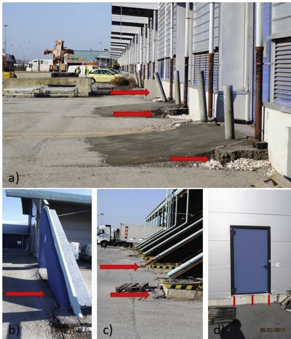
Fig. 2. Examples of damages induced by the subsidence in the of the freight terminal area.
