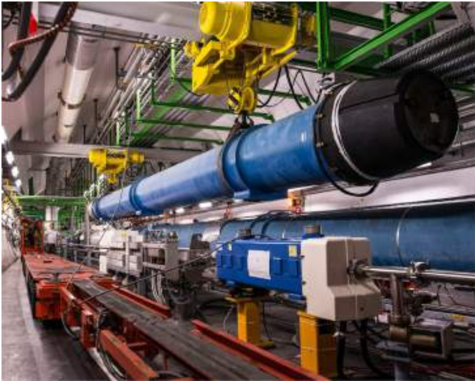
Fig. 5.13. Transfer of an LHC cryo-magnet between the transfer tunnel TI 2 (foreground/left, with the beam line arriving from the right) and the LHC main tunnel (background/right).
