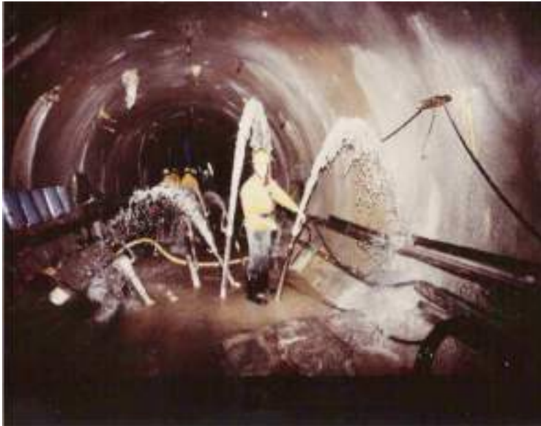
Fig. 4.10. Water inflows during LEP tunnel construction.
