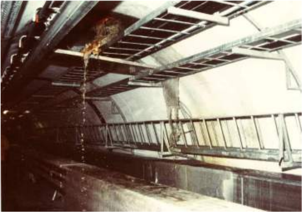
Fig. 4.11. Failure of tunnel concrete lining in 1990.
