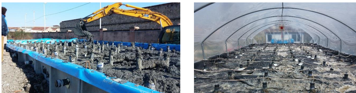
Figure 1. Left: filling of the basin with dredged sediments (February 2015). Right: plant installation completed (April 2015).
