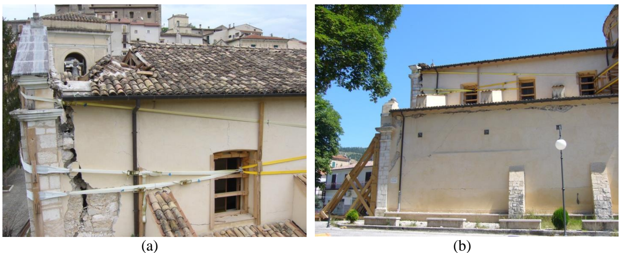
Figure 13. View from south of the façade mechanism at the top (a) and at the lower part(b).
