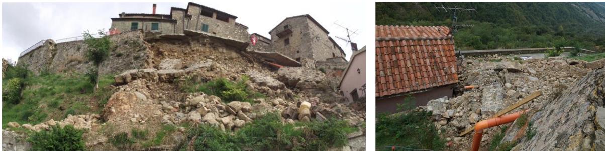
Figure 3: Collapse of the city walls in Cana di Roccalbegna (October 5, 2013). On the left: the collapse seen from below; on the right: the debris near the building below the wall.
