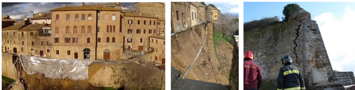
Figure 4: The collapse of the city walls of Volterra (January 31, 2014).
