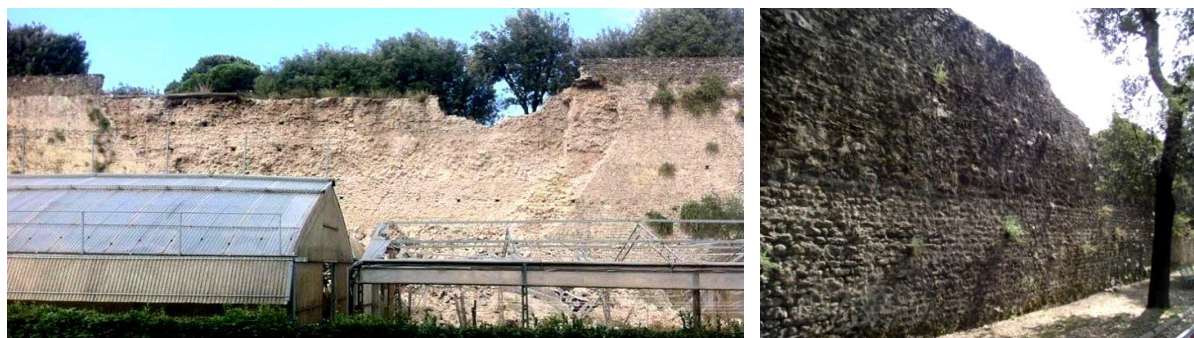
Figure 1: Collapse of the city walls of Pistoia (September 19, 2011). On the left: the failure seen from the outer side; on the right: the failure seen from the city centre.
