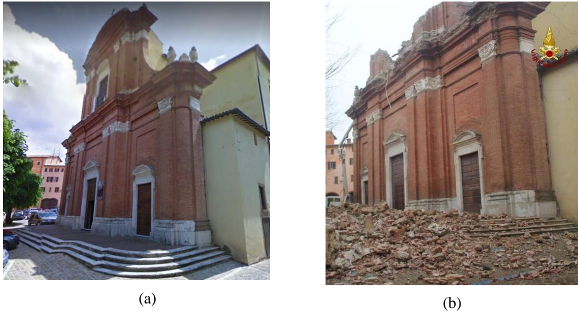
Figure 6: Case of study: San Filippo Neri's church in Camerino (Macerata): main façade before (a) and after (b) collapse.
