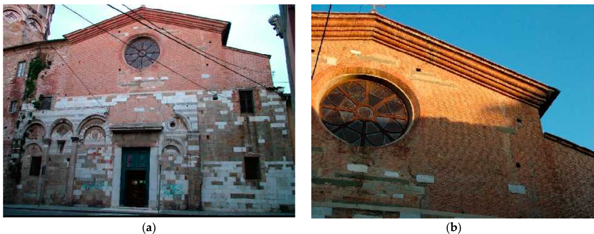
Figure 17. The crack pattern on the main façade: (a) general view; (b) detail.
