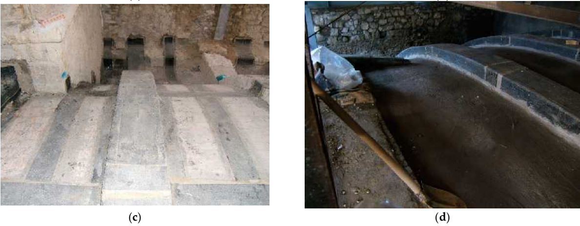
Figure 5. Composite strengthening of a partly collapsed ribbed barrel vault: (a) detail of the collapsed part; (b) reconstruction of the collapsed part; (c) detail of composite reinforcement; (d) detail of the completed intervention.
