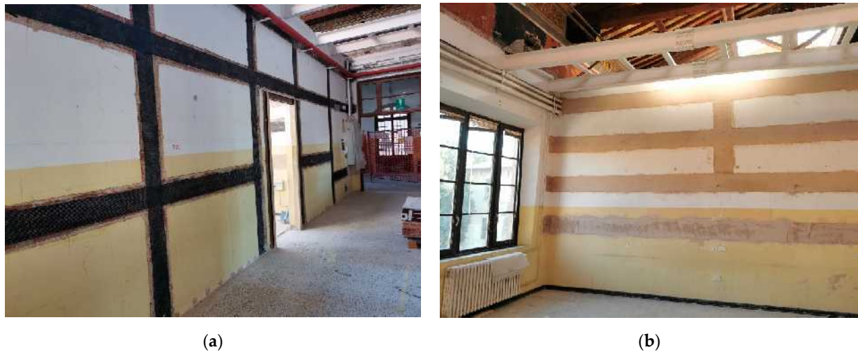
Figure 6. Composite intervention to avoid overturning of partition walls: (a) application of the composite reinforcement; (b) detail of the completed intervention.
