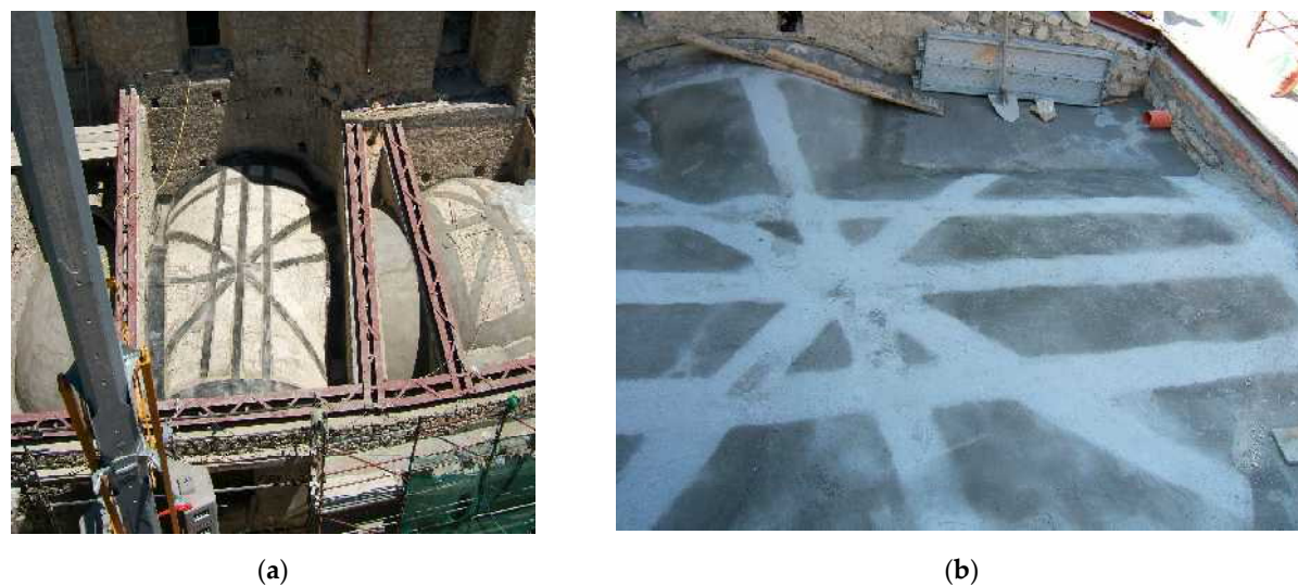
Figure 3. Composite strengthening of a cross vault: (a) detail of the composite reinforcement; (b) detail of the completed intervention.
