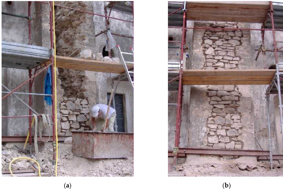
Figure 7. Application of the indentation technique to the strengthening of a parastas: (a) during the intervention; (b) at the end of the intervention.
