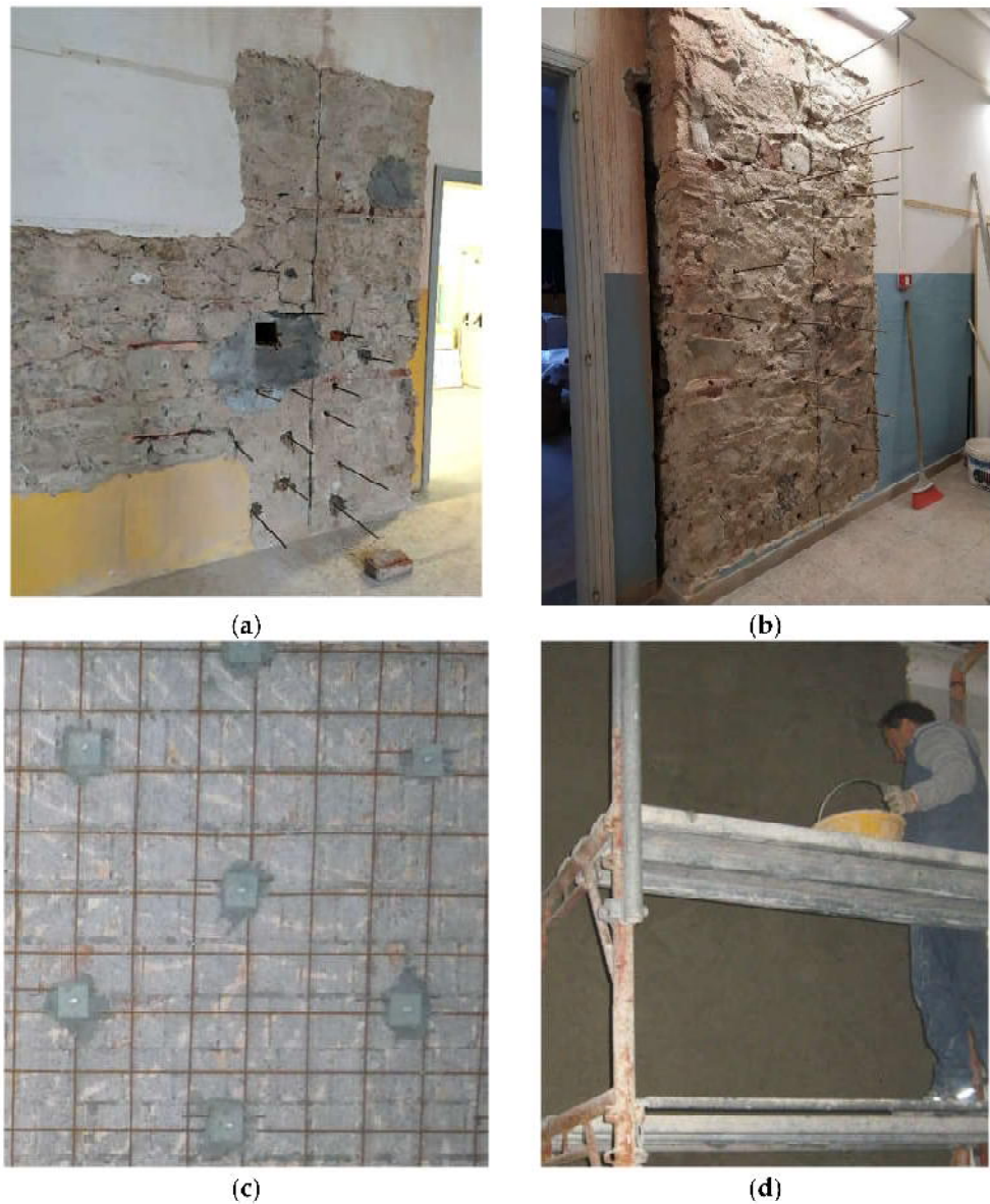
Figure 6. Strengthened technique adopted to restore the tested walls: repair of cut and cavity (a), insertion of threaded or reinforcing steel bars (b), application of the reinforcing steel mesh (c), and final grouting of the concrete layer (d).
