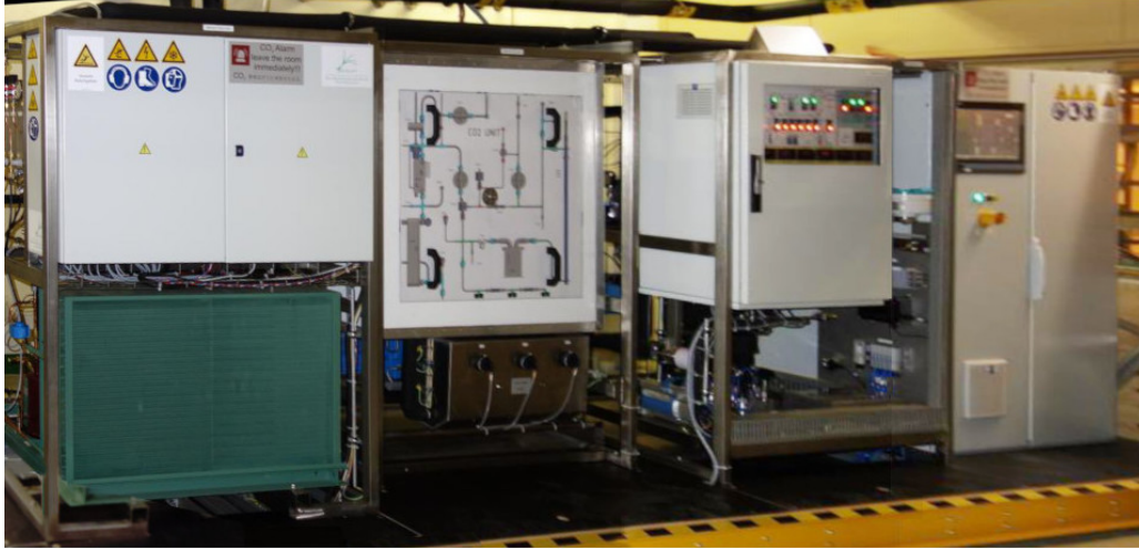
Figure 75. The IB Belle cooling plant. The four chassis from left to right are for the R404A refrigerator, the CO 2 pumps and tubing, the accumulator, and the control unit. In total, the cooling plant occupies a 6 \times 1.5 \times 2 \text{ m}^3 volume.
